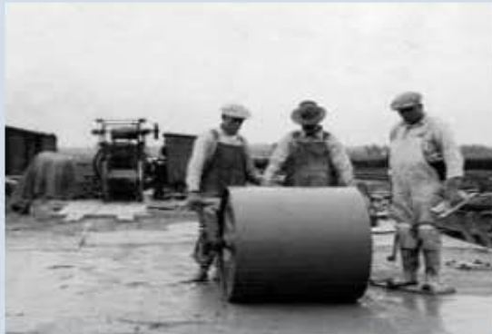
Early 1940s: The first RCC pavement in North America is an airport runway constructed in Yakima, Washington.
