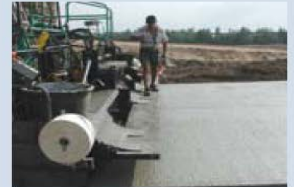
2000s: RCC pavements gain popularity for constructing low- to moderate-traffic streets and secondary highways.
